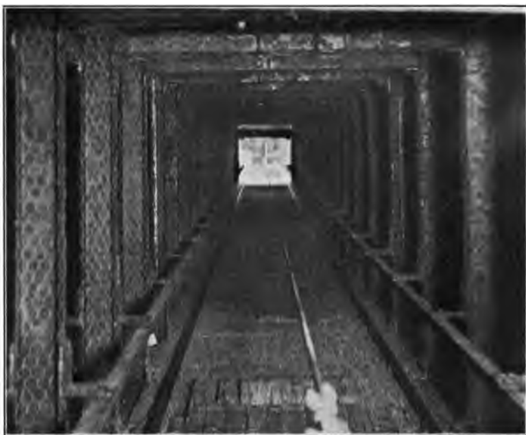
VIEW LOOKING UP "A" SHAFT SHOWING COMPLETED GUN-CRETE WORK ABOVE. RE-INFORCING SET BELOW BUT NOT CONCRETED YET
